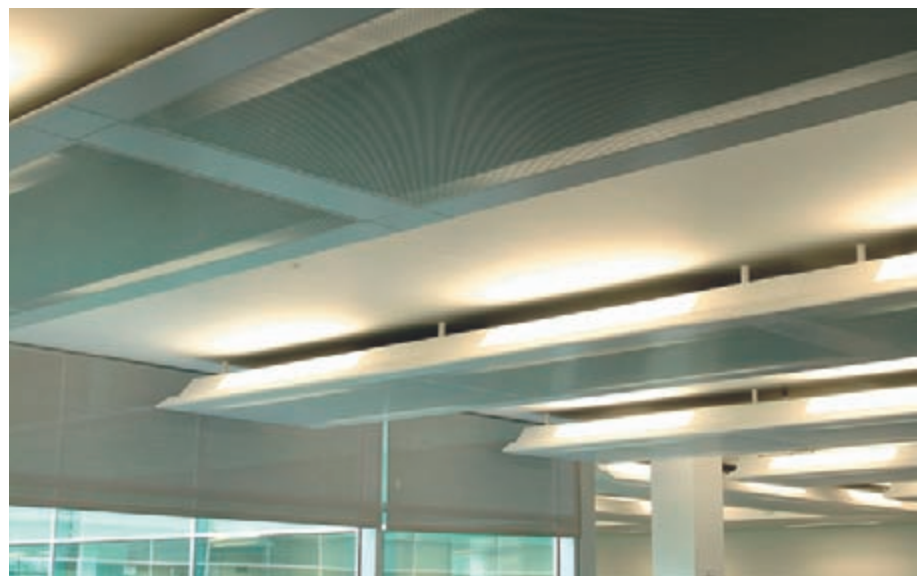
Chilled beam system showing the use of uplighting to illuminate the soffit, courtesy of Frenger Systems Limited.
