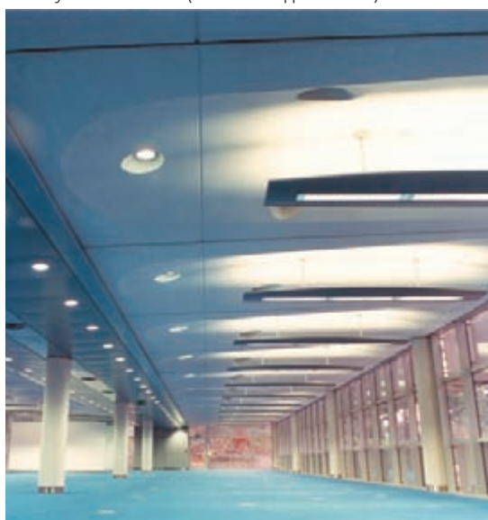
Toyota GB Headquarters: interior (left), precast concrete soffit unit (right), courtesy of Trent Concrete (Architect: Sheppard Robson).
